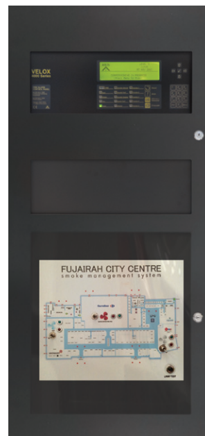
FIRE ALARM PANEL WITH SMOKE MANAGEMENT SYSTEM
