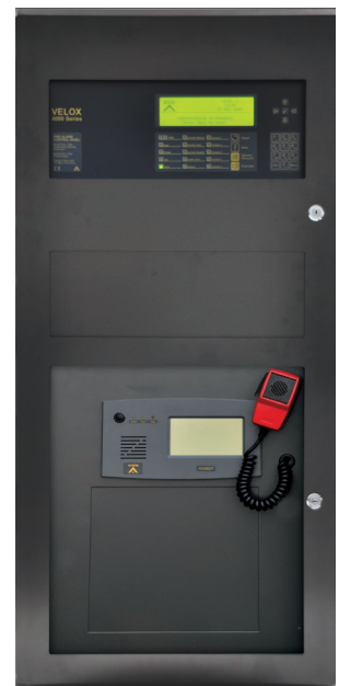
FIRE ALARM PANEL WITH PSSAS
